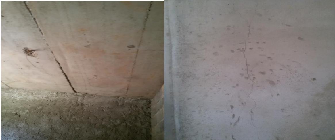
Figure 4.2 Fissurations du béton
