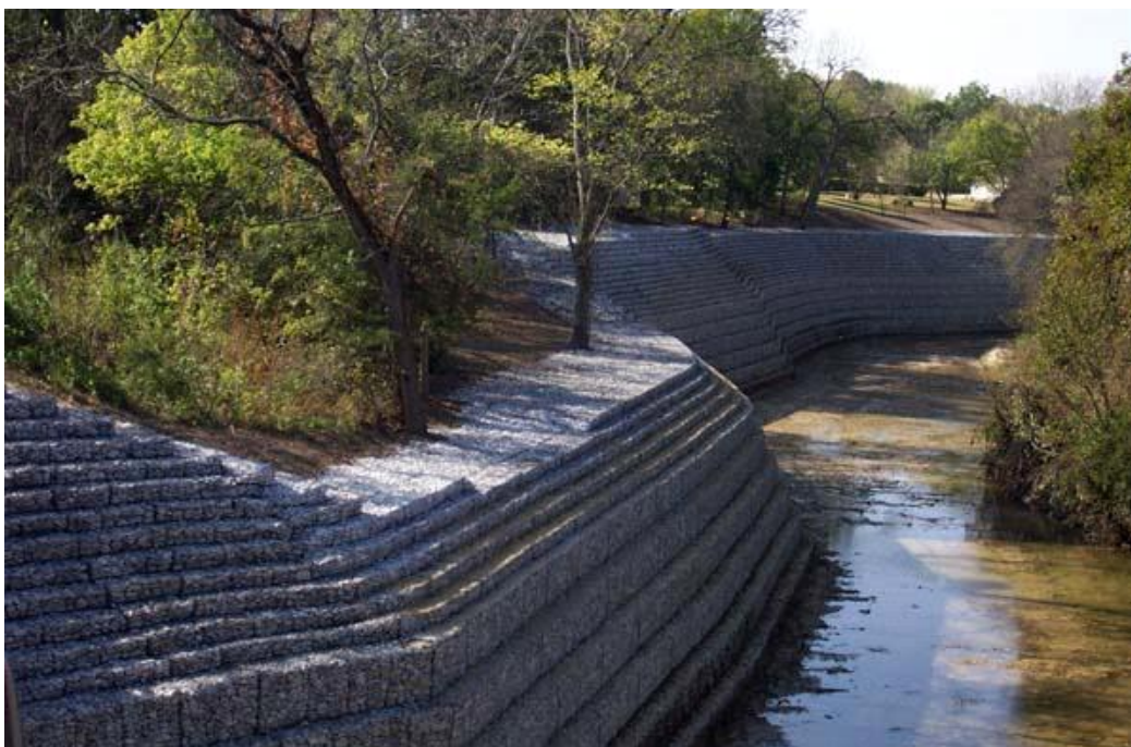
Fig.VI.12: renforcement par gabions (Water And Soil Erosion Preventing Gabion Baskets / Boxes with Hexagonal Wire Mesh)
